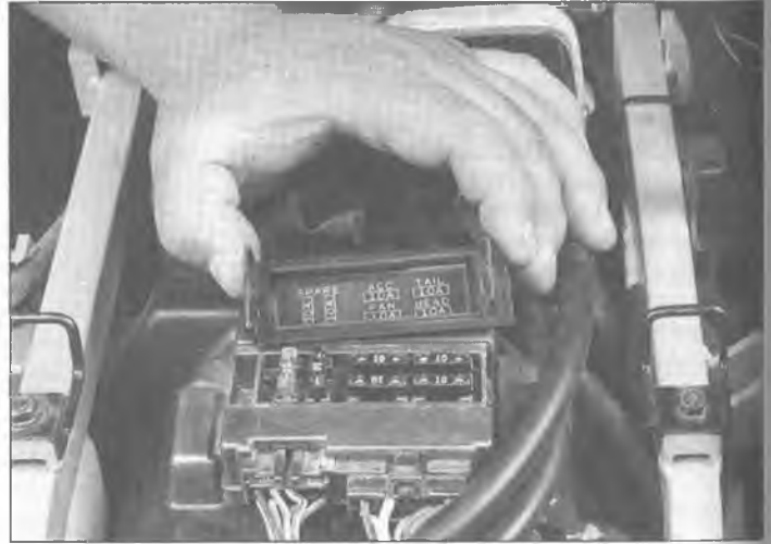
5.1b This junction box is on an E model, under the seat, on top of the rear fender/mudguard
