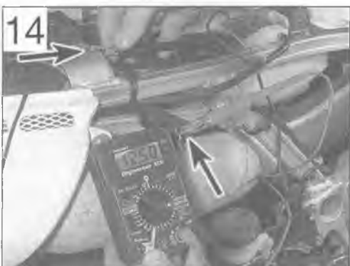
14 Checking for voltage at the rear brake light power supply wire using a meter . . .
