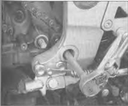
5.18a Hold the bolt on the left side of the frame and unscrew the lower rear engine mounting nut
