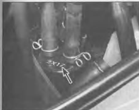
7.3 The liquid/vapor separator (arrow) is on the right side, below and in front of the IC igniter
